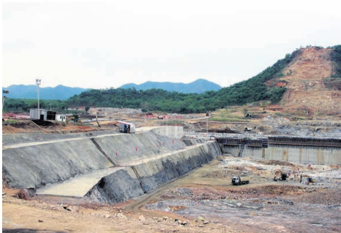
In this June 28, 2013 file photo, construction work takes place, at the site of the Grand Ethiopian Renaissance Dam near Assosa, Ethiopia.
